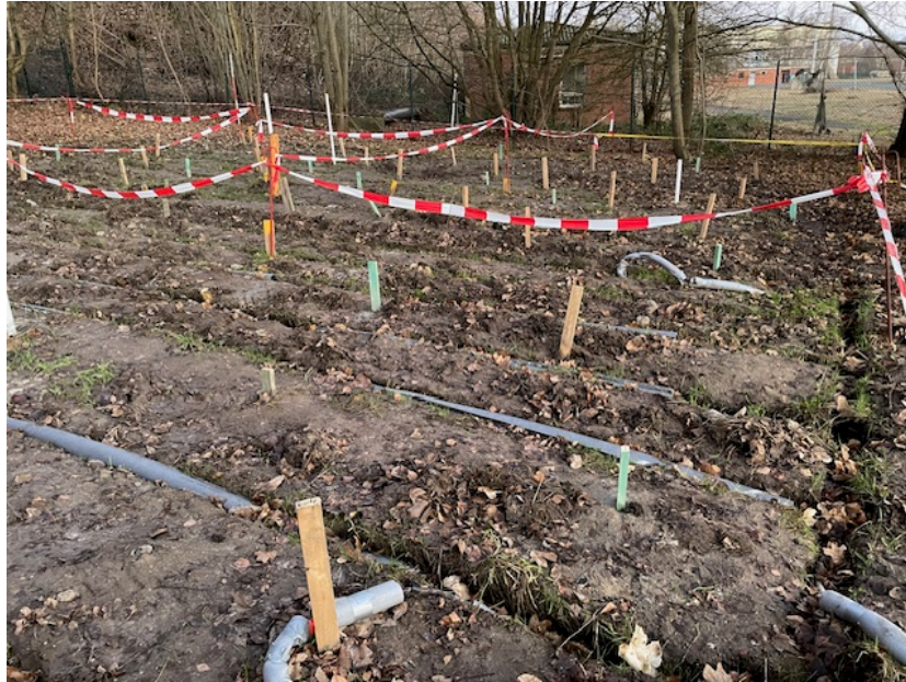
Figure 1: Photograph of the pilot installation with drainage trenches
