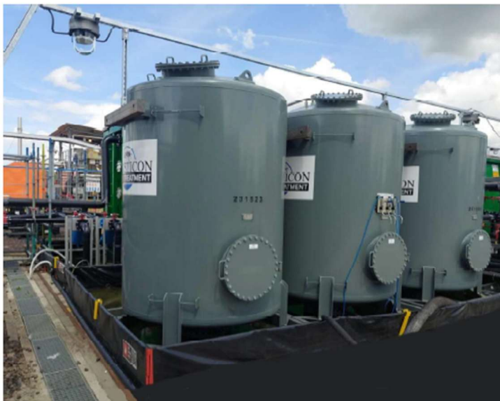
Fig. 2 IEX resin vessel cascade for the adsorption of short-chain PFAS at Chemours in Dordrecht, South Holland (The Netherlands) Photo: Chemours Dordrecht with courtesy of Logisticon Water Treatment
